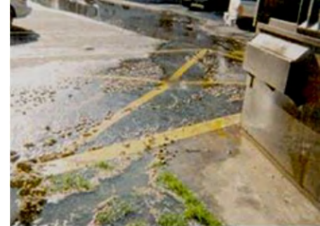
Figure 3: A FOG related SSO in a parking lot.
