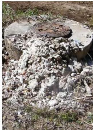
Figure 42: Grease interceptor overflow.
