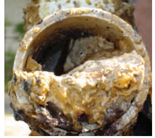
Grease clog inside a pipe.
