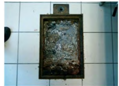
Figure 43: Grease trap overflow is a hazard to kitchen employees.
