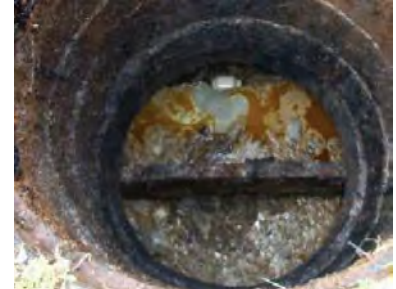
Figure 34: Too short outlet tee allows short-circuiting.
