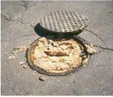
Figure 22: Interceptor filled with grease to the top.
