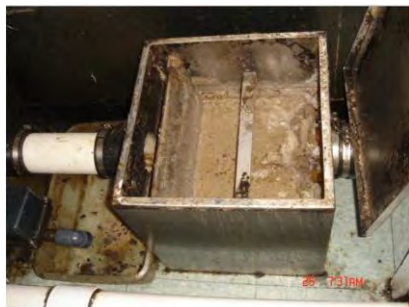
Figure 16: Grease trap installed above ground.
