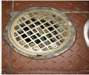
Figure 30: Debris in the floor drain (floor was not swept before mopping).
