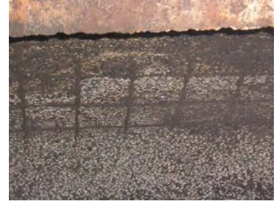
Figure 37: Exposed re-bar in a corroded concrete interceptor.
