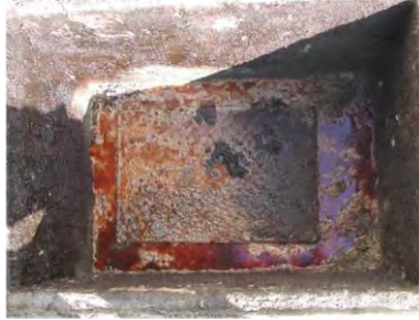
Figure 33: Grease interceptor not working.
