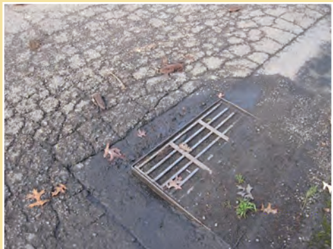
Standing water due to clogged drains can damage pavement.
