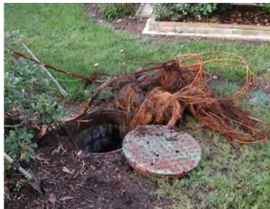
Figure 35: Roots removed from the grease interceptor (root intrusion can completely clog the interceptor).
