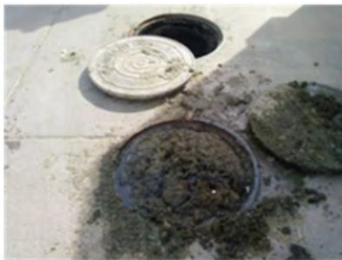
Figure 41: Grease interceptor completely full. Heavy lids can be lifted up under pressure and grease start overflowing.
