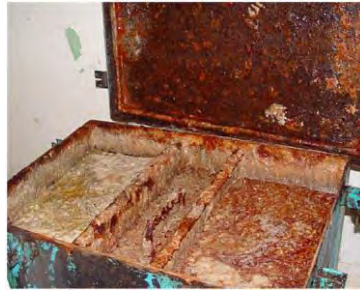
Figure 36: Severely corroded metal grease trap (these traps are highly prone to corrosion).
