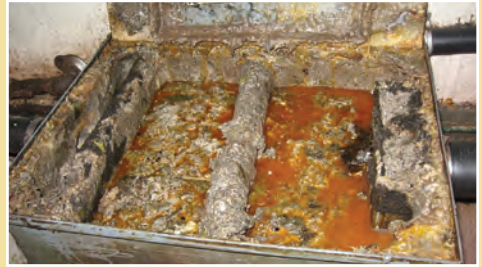
Interceptor too full of FOG and not maintained properly; will cause building sewer problems.
