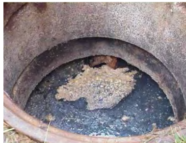
Figure 39: Missing outlet tee allows floating FOG to escape into the sewer system.
