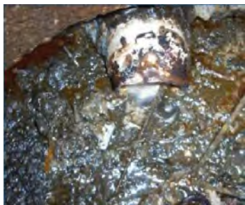
Figure 38: Missing inlet tee allows FOG buildup in front of discharge pipe.
