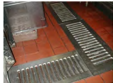
Figure 9: Floor drain screen.
