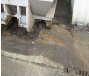
Figure 32: Waste leaks in the garbage and grease recycle storage area.
