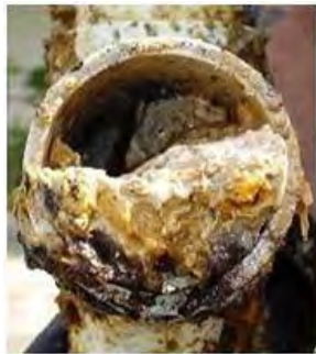
Figure 1: FOG deposit clogging the sewer pipe.
