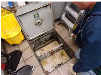
Figure 17: Grease trap installed flush with the floor (an in-floor trap).
