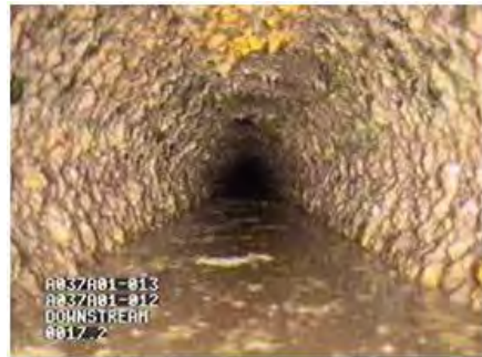
Figure 2: FOG accumulated on the wall of sewer pipe.
