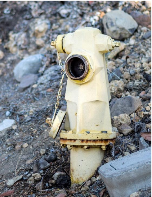
Figure 1. Opened fire hydrant allowing air to enter the system.
