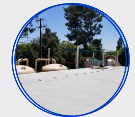
City of South Pasadena, California Graves Reservoir Replacement and Wellhead Water Treatment Grand Reservoir Replacement Project
