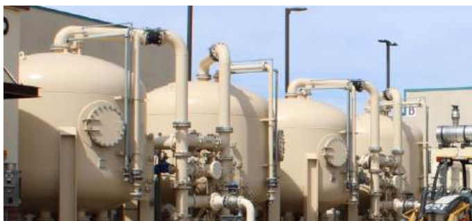
East Orange County Water District Treatment Facility
