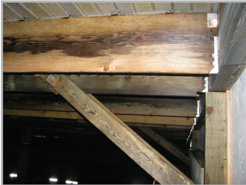
Photo B.8 Peters Canyon Reservoir Typical Purlin and brace at Perimeter Wall
