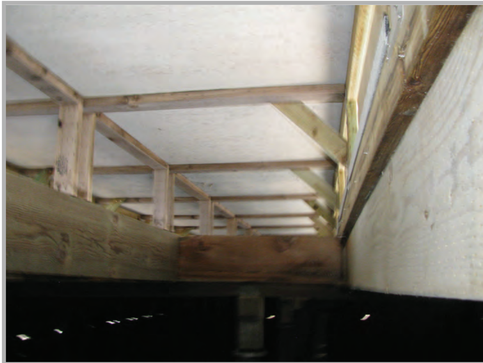
Photo B.10 Peters Canyon Reservoir Typical Framing at Central Vent
