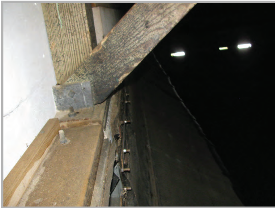
Photo B.9 Peters Canyon Reservoir Typical Brace Bottom Connection at Perimeter wall
