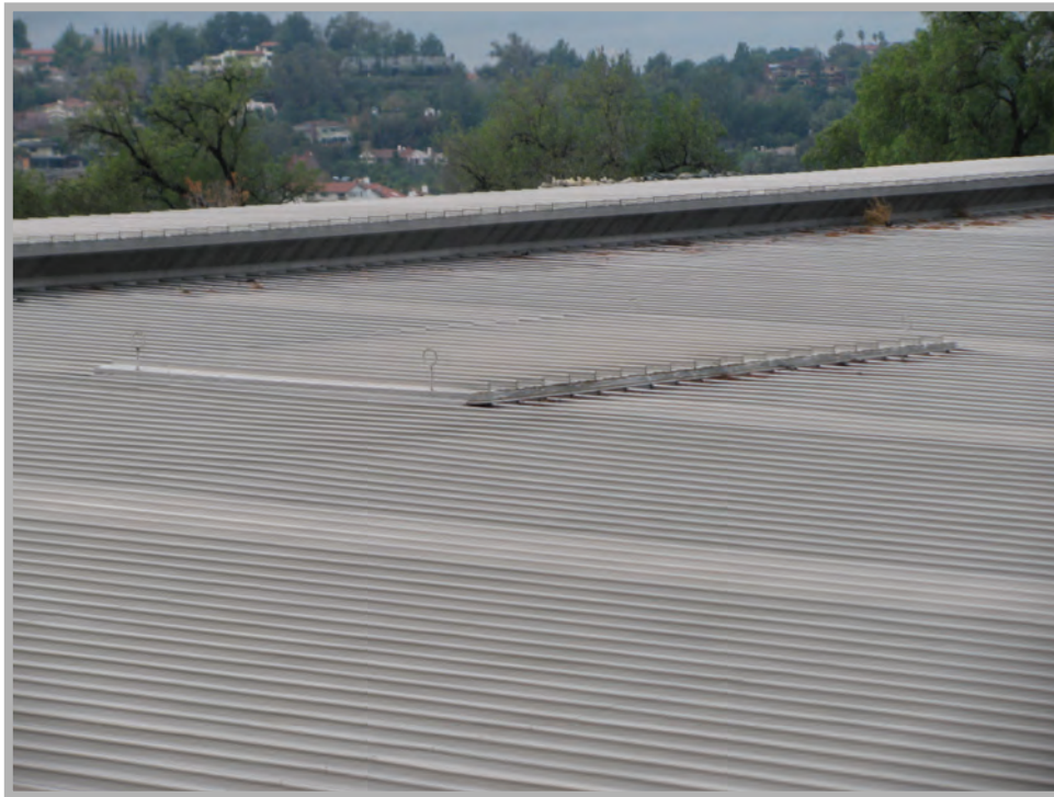
Photo B.3 Peters Canyon Reservoir Roof Central Vent
