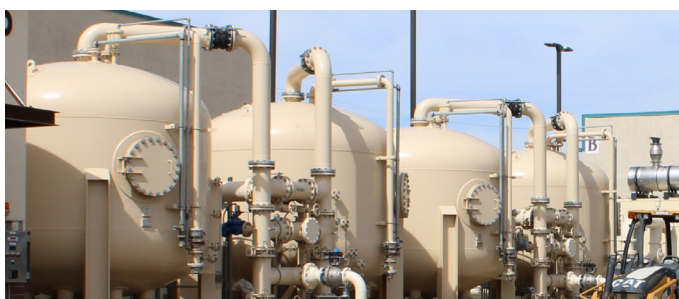
East Orange County Water District Treatment Facility
