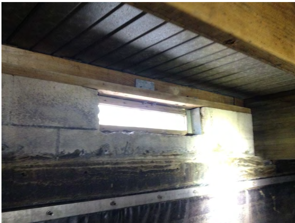
POST CONSTRUCTION INSTALLED VENT
