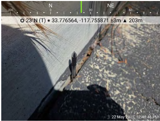
Close up view: minor edge cracking observed
