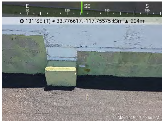
Far view: Corner tale crack monitor B" relative to pilaster
