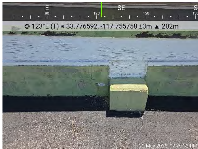
Far view: Corner tale crack monitor C" relative to pilaster
