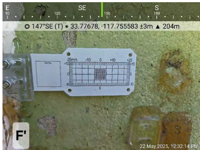
Close up view: Corner tale crack monitor F" with one side detached
