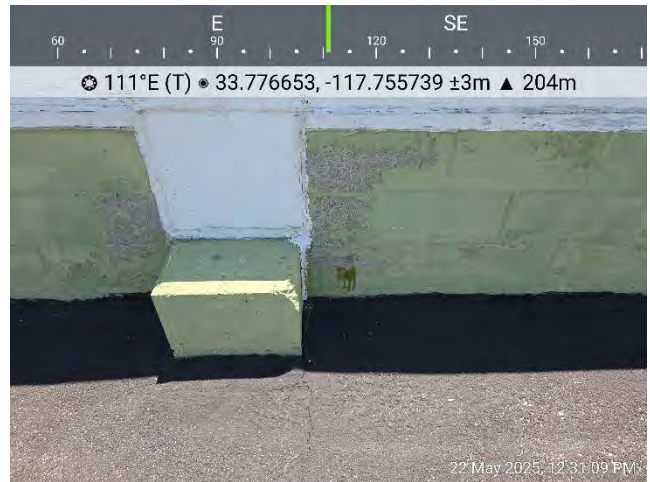
Far view: Portion of corner tale Crack Monitor A" missing
