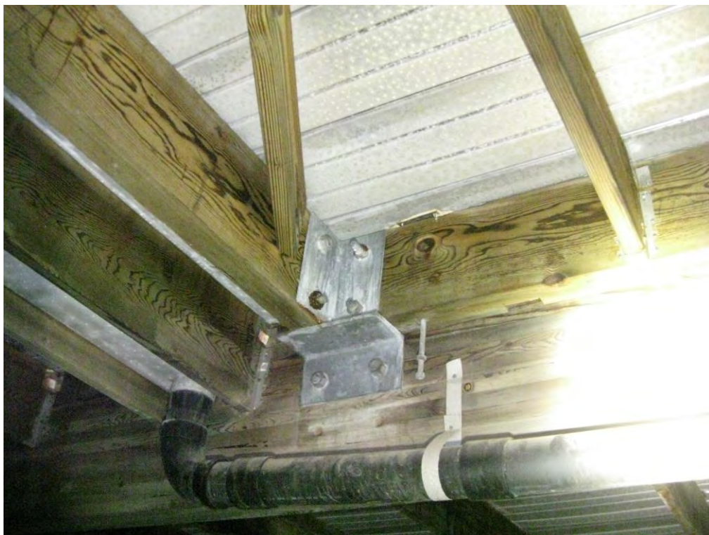
COROSION ON LIFT OUT ROOF PORTAL
