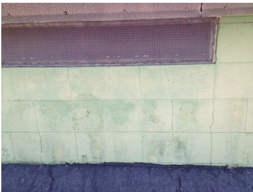
THERMAL SHRINKAGE EFFECTS ON SOUTH WALL 2
