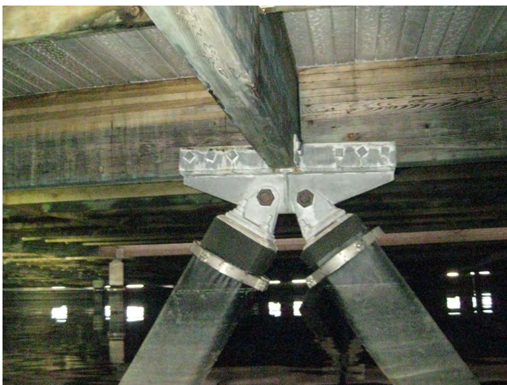
TYPICAL BRACED FRAME CONNECTION (CORRODED NUTS AND BOLTS)
