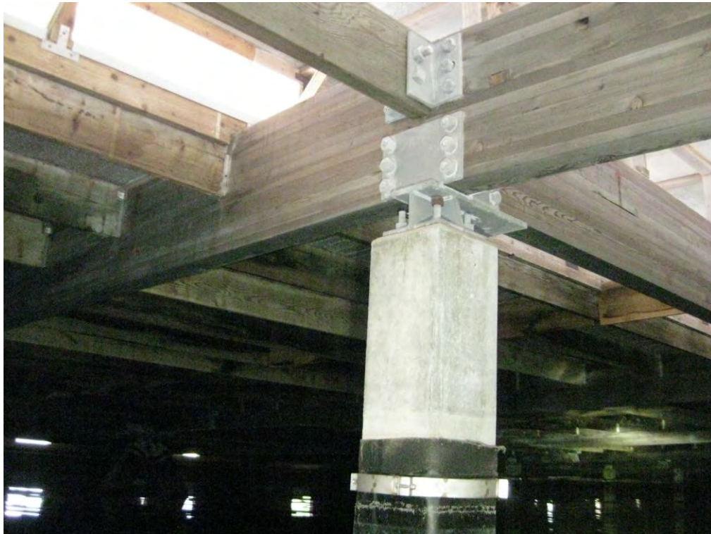
COLUMN WITH LOOSE NUT ( NON-GALVANIZED)
