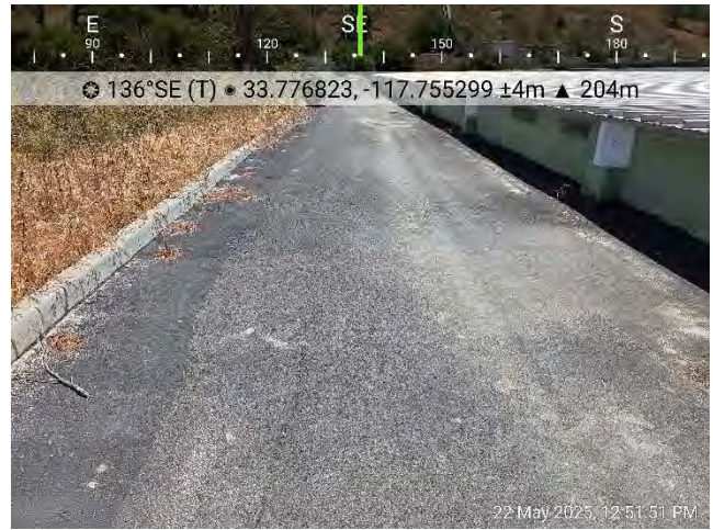
view: Asphalt surface along the North end of the site. Low severity cracking observed
