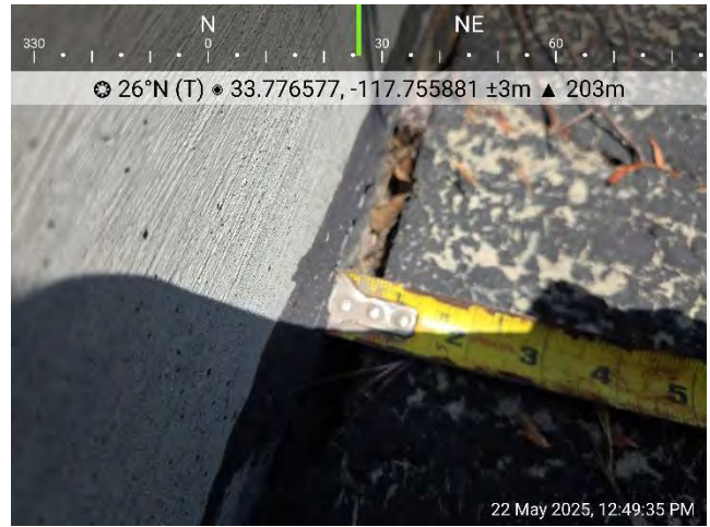
Close up view: minor edge cracking measured. Less than 1"
