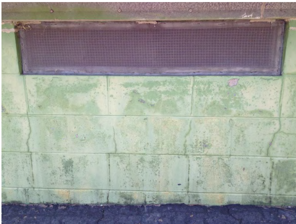
THERMAL SHRINKAGE EFFECTS ON SOUTH WALL 1
