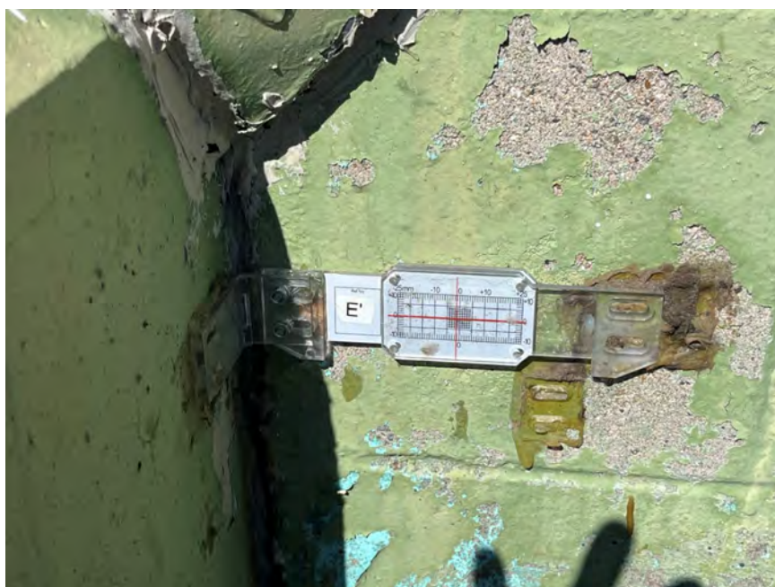
Figure 22 Reservoir Crack/Movement Monitoring
