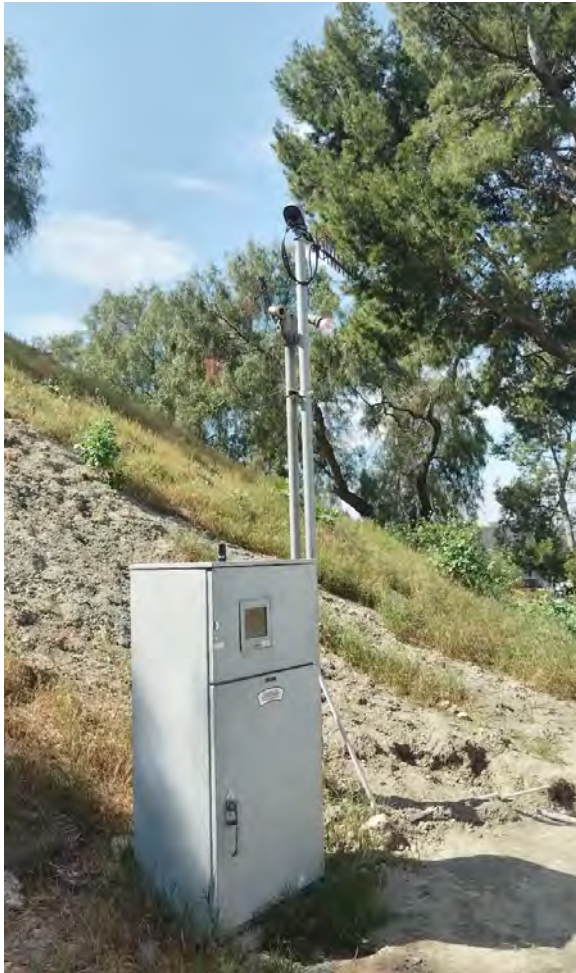
Figure 49 Existing SCADA Panel
