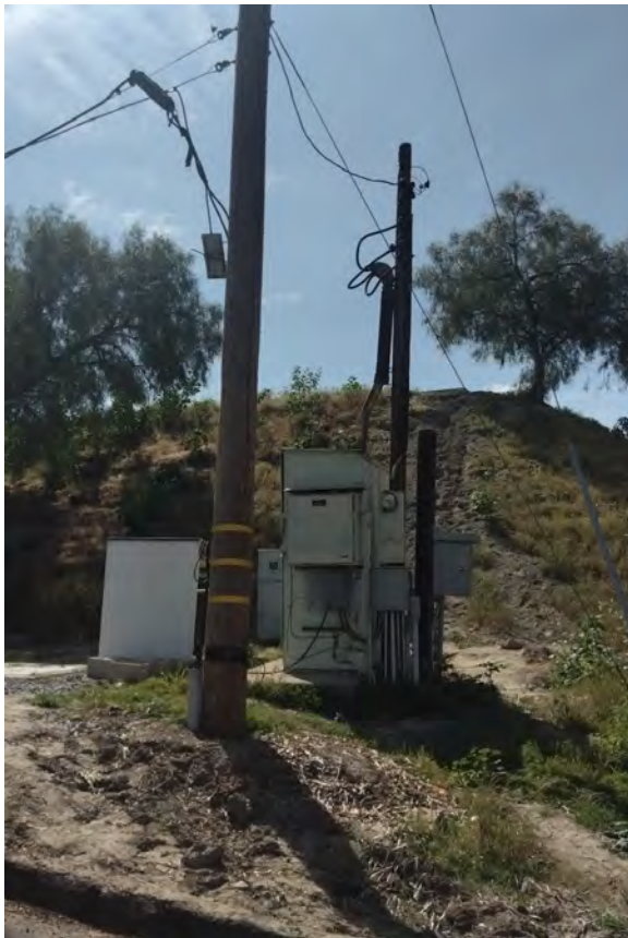
Figure 48 Existing SCE Electrical Source
