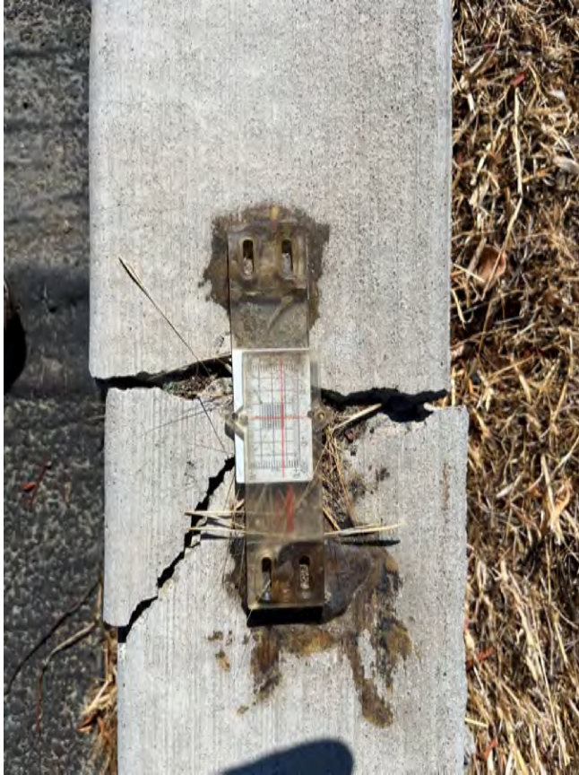
Figure 23 Curb Crack/Movement Monitoring
