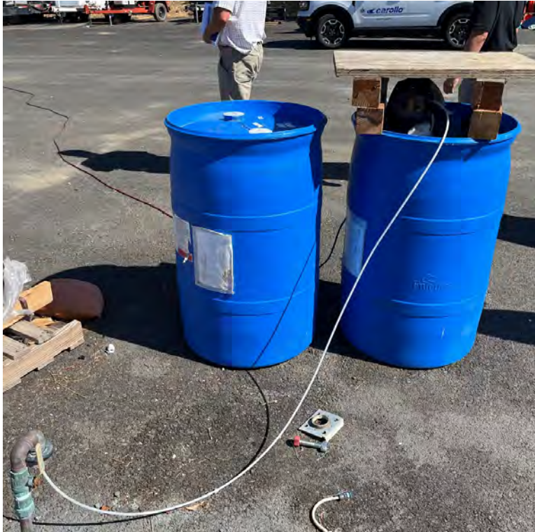
Figure 50 Temporary Hypochlorite Dosing System at Peters Canyon Reservoir
